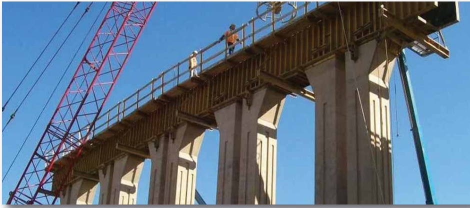
Construction has begun on Chisholm Trail Parkway. Pictured is work on one of the early segments, a bridge over the Davidson rail yard. Photo: NTTA
